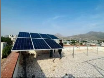
3.24 kw on grid solar system
