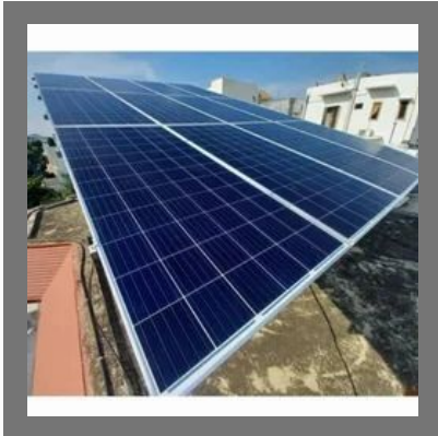
30kW Solar Power Plant
