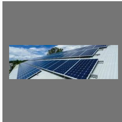
10 KW Solar Rooftop Power Plant
